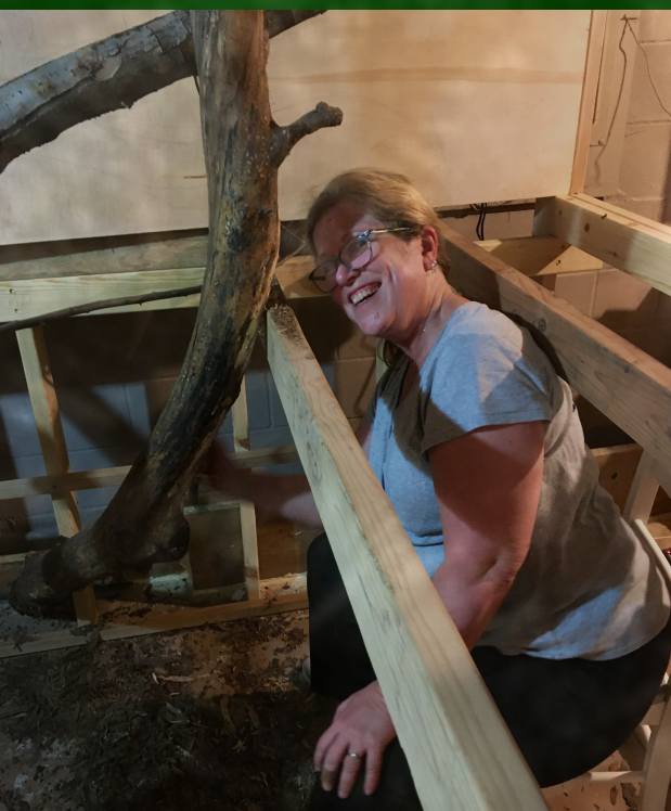
Helped build a club house for the girls in the basement, getting ready for the Minnesota winter
