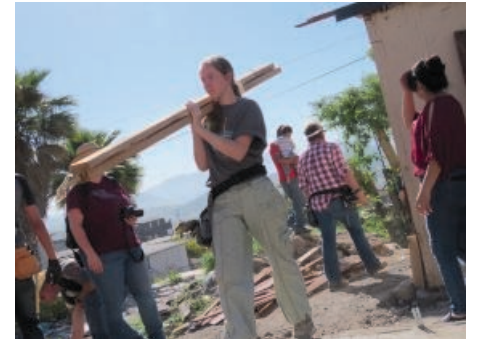
Here is Bekah and her group helping build 2 of the 4 houses in Mexico.
